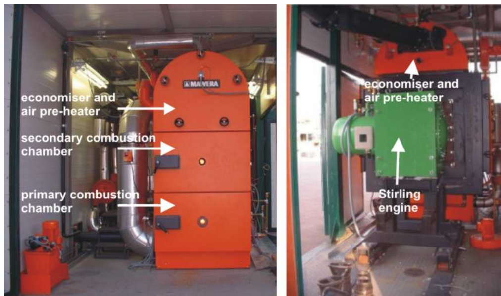
Figure 7: Pictures of the small-scale CHP pilot plant with a 35 kW el Stirling engine
