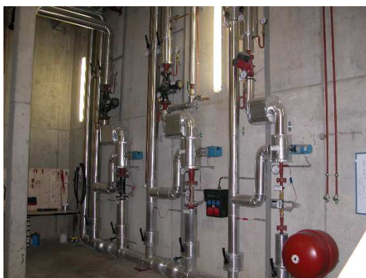
Hydraulic control loop in the heating plant
