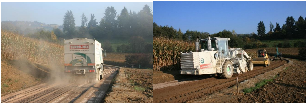
Application of wood ash with a spreader (left), mixing with the soil to be stabilized by a rotary hoe (right)
