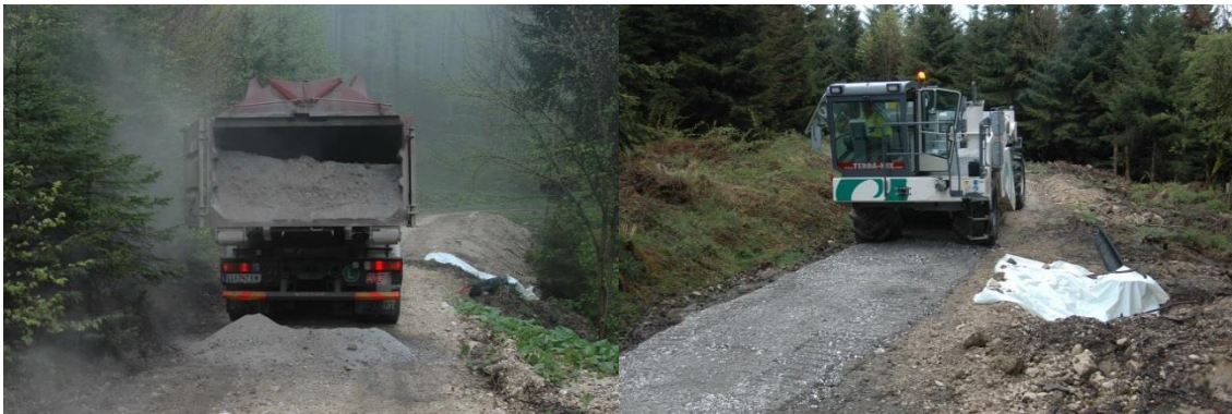
Application of wood ash by tipping the ash on the road (left), mixing with the soil to be stabilized by a rotary hoe (right)
