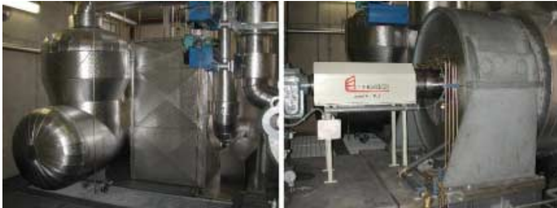
Figure 5: View of the evaporator (left picture), the turbine and the generator (right picture)
