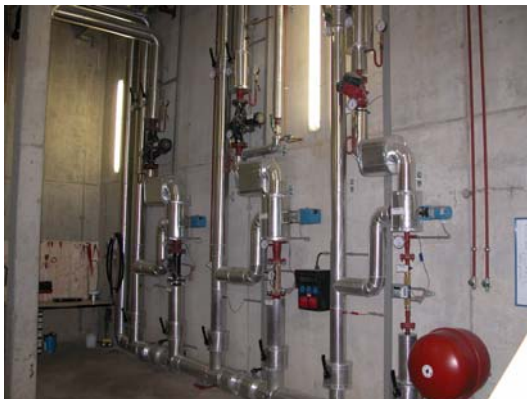
Hydraulic control loop in the heating plant
