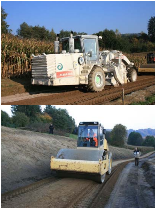
Figure 8: Mixing of the binder with a rotary hoe and subsequent compacting with a roller compactor
