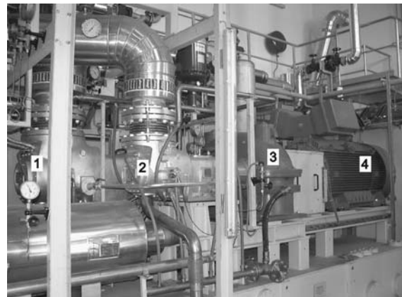
Figure 8: Screw-type steam engine of the biomass CHP plant in Hartberg (net nominal electric capacity: 710 kW el )
