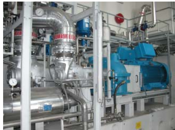
Screw-type steam engine (730 kW el ) at the biomass CHP plant Hartberg (A)
