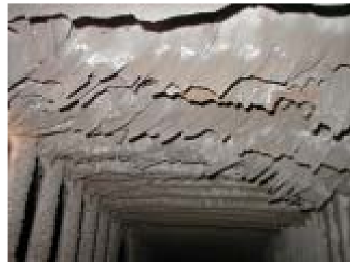
Hard super heater deposits in a waste wood fired boiler
