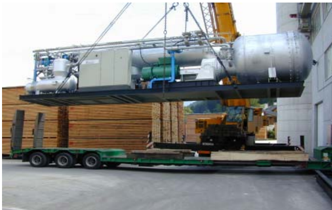
ORC module in container design (400 kW el ) at ist delivery at the CHP plant
