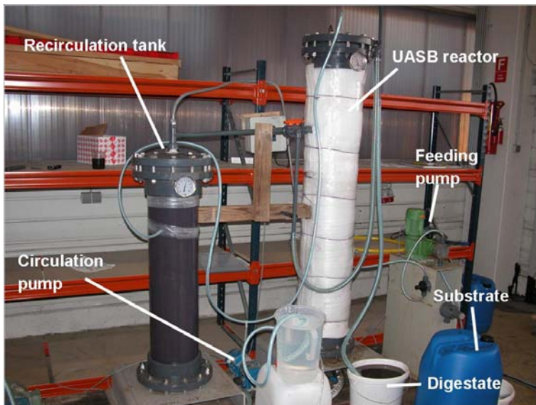
UASB pilot plant (UASB: upflow unaerobic sludge blanket)
