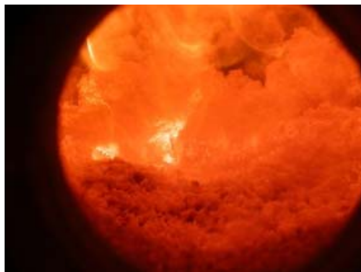
View into the furnace of a pilot-scale grate-fired combustion plant during test runs with a new biomass fuel in the course of combustion plant development
