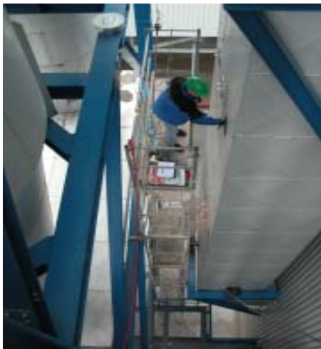
Measurement campaign at a real-scale combined heat and power plant
